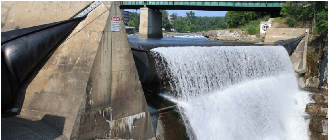
Water-filled Rubber Gate (Hydropower)
